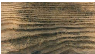
Mold infestation on spruce after one year of external weathering in a moist climate
